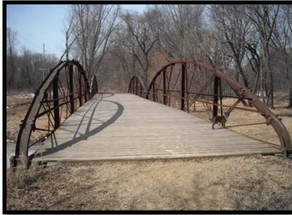
#3 - McGilvary Bridges*—This photo is of one of seven bridges located in the Van Loon Wildlife Area, also known as the McGilvary Bottoms. These bridges were constructed to aid in spanning the maze of sloughs and channels in the bottom. Today, there are five steel bowstring arch truss bridges, built between 1905 and 1908. The bridges were listed on the National Register of Historic Places in 1980, and McGilvary Road is designated as Rustic Road #64.
