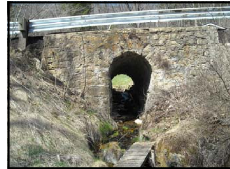
#6—Schmaltz Road Bridge, ca. 1930's. This stone bridge is located northeast of the intersection of STH 14/61 and CTH M on Schmaltz Road in the Town of Greenfield. It was made of locally harvested stone and constructed by the CCC established during the Great Depression.
